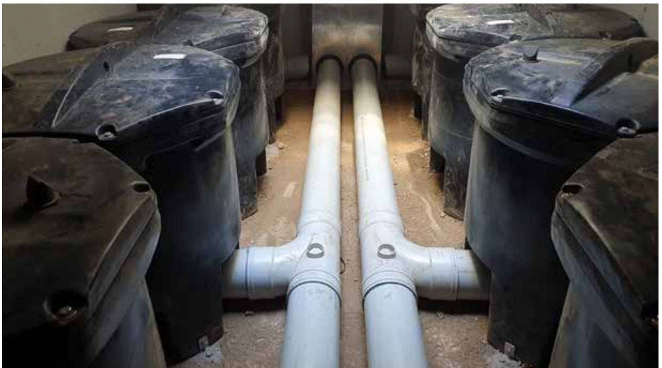
Figure 1 - SPELFilters in a concrete chamber / vault
